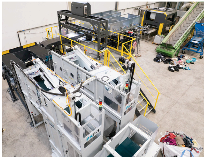
Picvisa's Ecosort sensor-based systems are installed at various sites in Europe. Image: Picvisa
